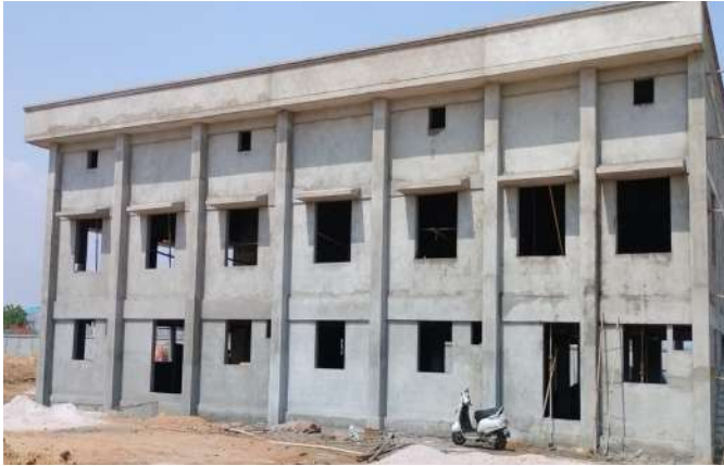
HT_LT_VFD Building Mithirohar
