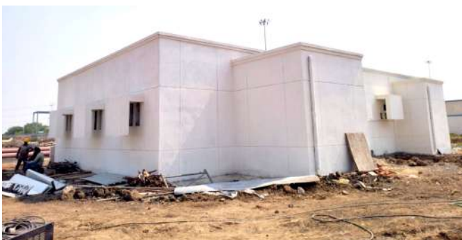
Control building Dumad
