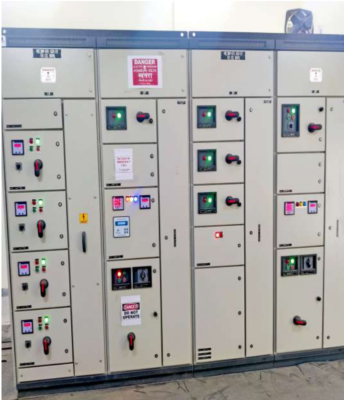
LT PMCC panel at IOCL Delivery Station Bhopal ▼
