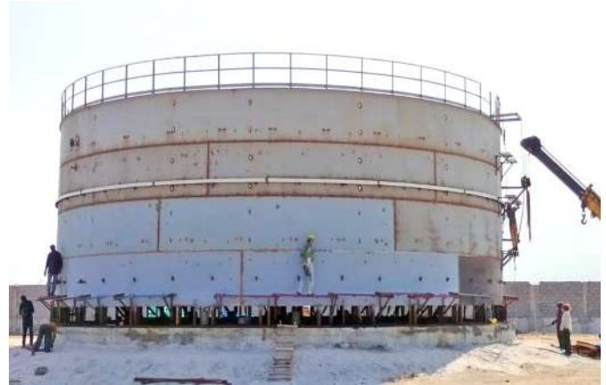
Fire water tank mithirohar
